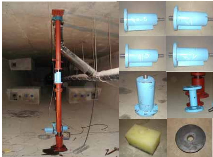
Figure 5. Installed dampers for the reduction of local vibrations and adopted devices
