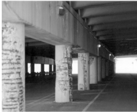
Figure 1. Damaged columns of a highway bridge.
