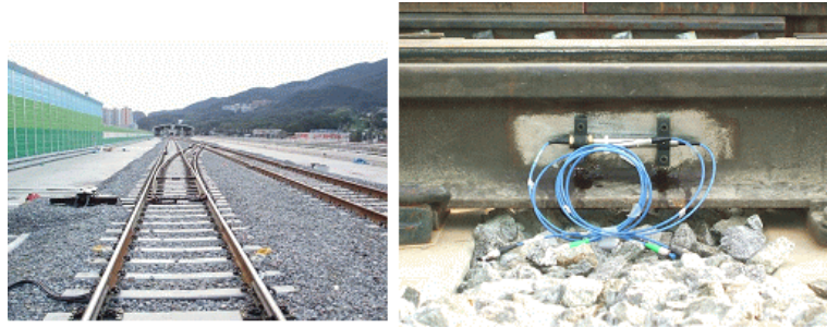
Figure 7. Track Behavior Monitoring Using Optical Fiber Sensors between Pyeongnae-Hopyeong Stations (Korea)
