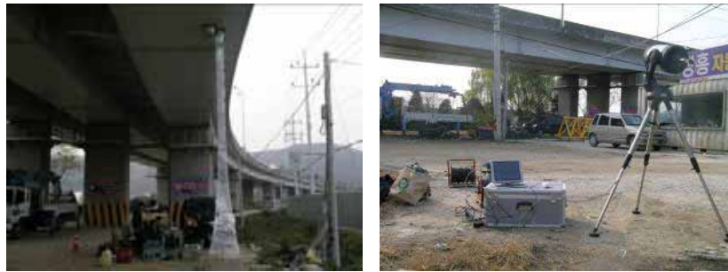
Figure 8. Contact and non-contact sensors installed on Jangheung Viaduct
