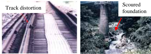
Figure 3: Site-situation of scour hazard in 1995
