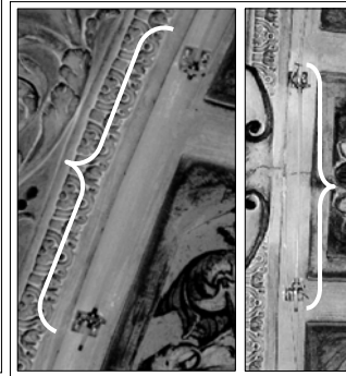
Figure 3. View of sensors installed in the vaults
