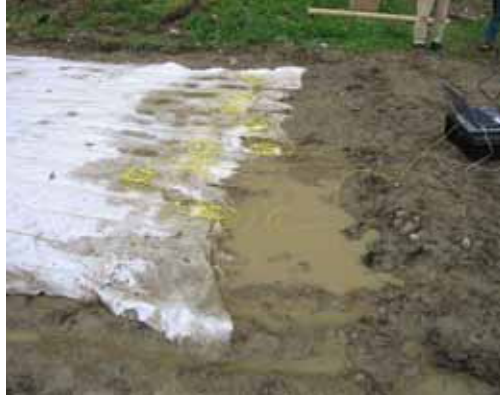
Figure 12. Sensor-based geotextile mat during installation on a construction site of a gravity dam in Solina/Poland.
