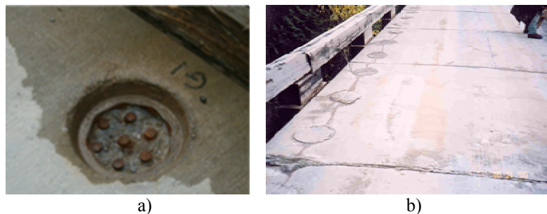
Figure 10. a) Exposed shear studs in one shear bulkhead; b) Longitudinal cracks between shear bulkheads
