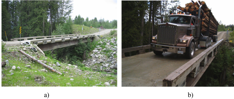
Figure 1. The Lindquist Bridge: (a) a view of the bridge; (b) a logging truck on the bridge.
