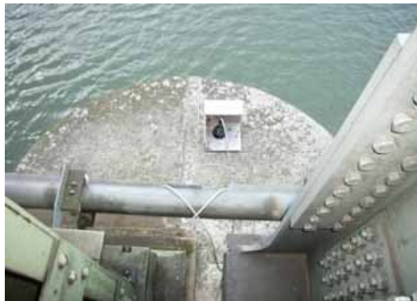
Figure 2. Sensor on the damaged pier
