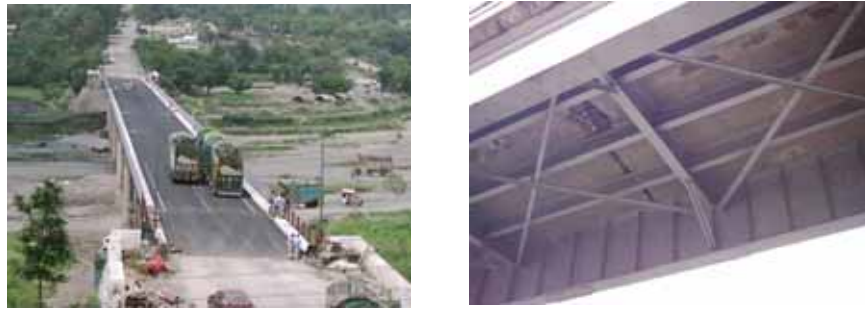
Figure 1. Ayub bridge: (a) global view, (b) underside view showing damages at joints
