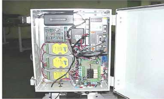
Figure 5. Programmable Logic Controller.
