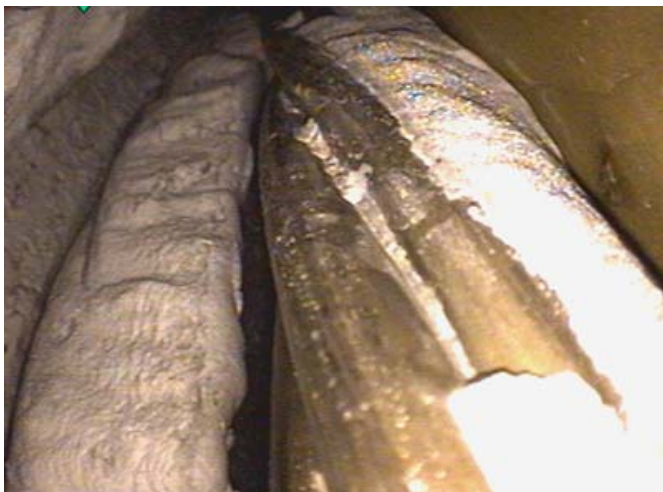
Figure 10. Voids inside the Bottom Duct (from Videoscope)
