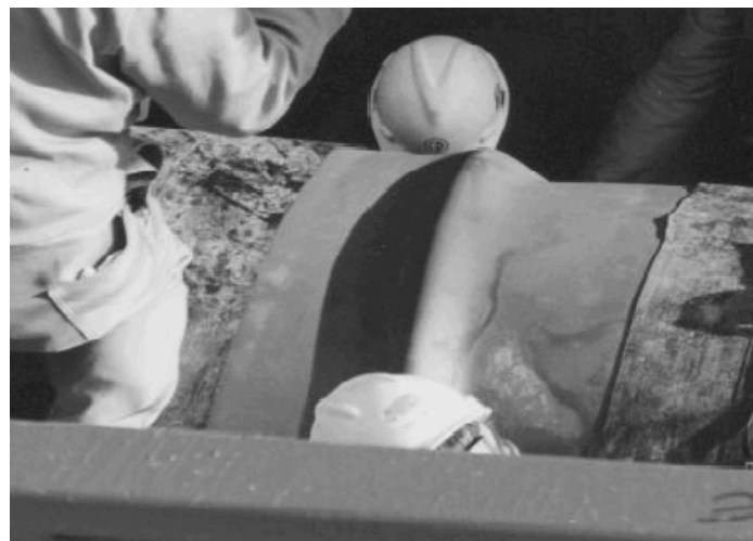
Figure 1. Pipe buckle and fracture
