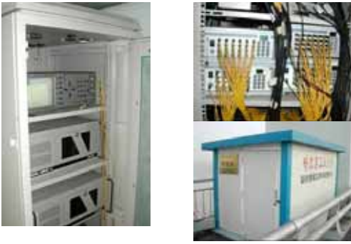
Figure 23. FBG monitoring system for Binzhou Bridge
