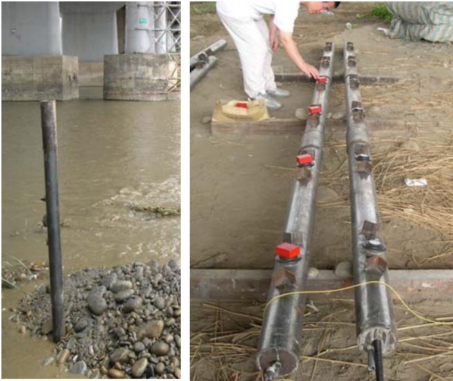
Figure 5. a) 4m-long FBG deformation sensor array inside pipe. b) Deformation sensor installed bridge footing.
