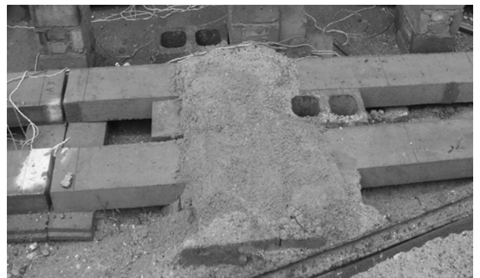
Figure 5. Corr_B corroded part covered with sands
