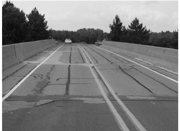
Figure 2. Bridge deck distresses and repair
