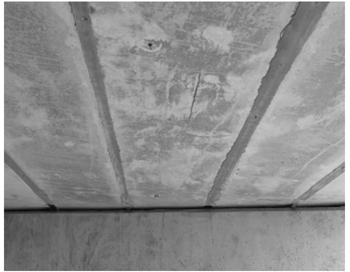
Figure 12. Moisture on beam soffits and post 1985 design shear keys
