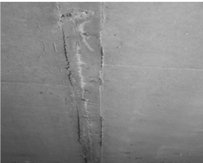
Figure 11. Efflorescence on the cracked post 1985 design shear key
