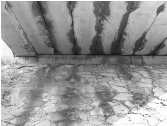
Figure 5. Moist beams, leaky joints, and moisture on stub abutment
