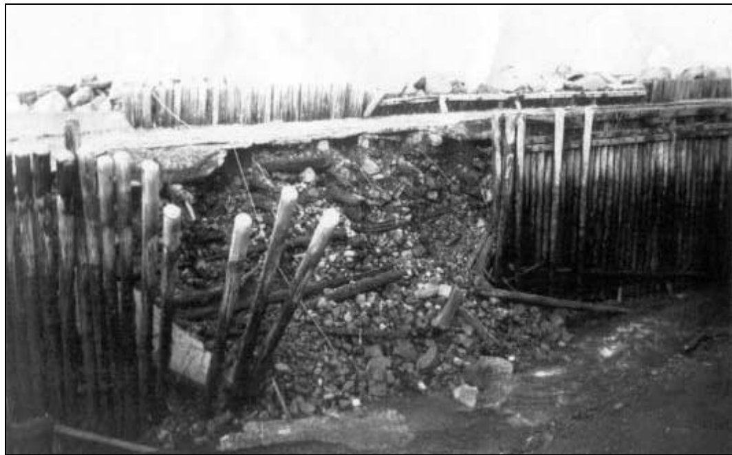
Figure 6.21 Failure of timber piles in Hall's Harbour
